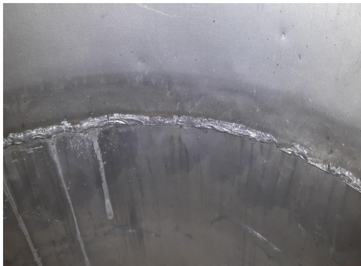
Figure 5: Improper surface finish [Inside view]
