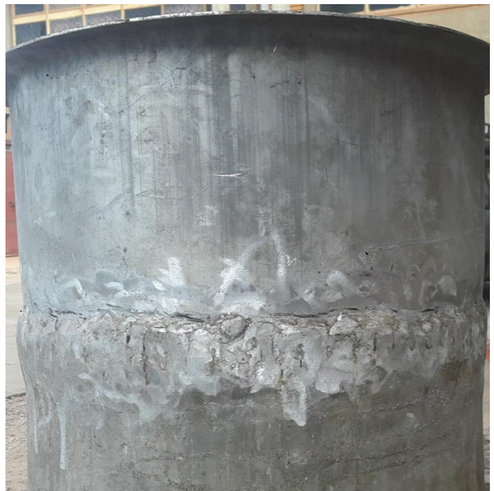
Figure 4: Improper surface finish [Outside view]
