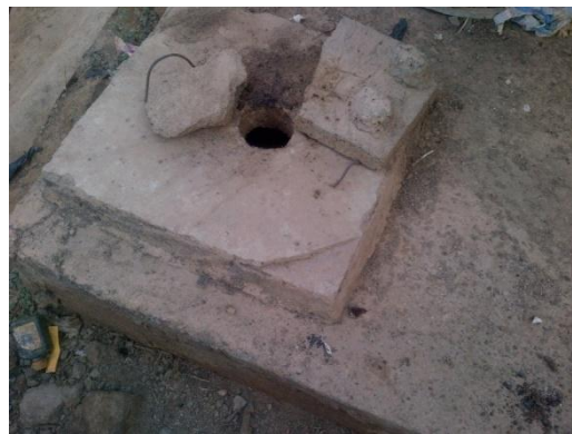
Plate 6: Condition of pit latrine in one of the slums
