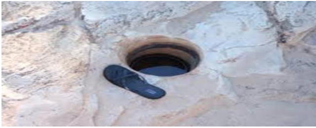
Fig 3: Original image considered for detection of Pothole
