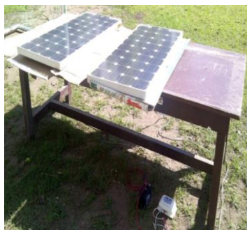
Fig. 5. Solar panel set-up
