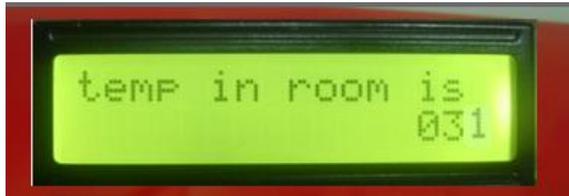
Fig17: Temperature display of room at the Transmitter Section
