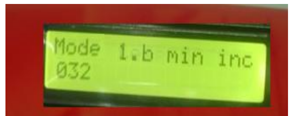
Fig 22: Display of Minimum temperature of the room set by the user at the Transmitter Section
