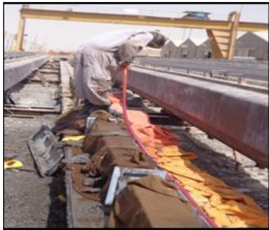
Figure (9) Casting of Concrete, Removed Forms from Beams Specimens and Curing by Burlap Sacks.
