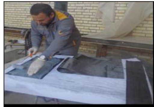
Figure (11) Cutting CFRP Sheet, Apply Epoxy on CFRP and Concrete, Placing CFRP on Concrete, and Eliminating Air Bubble, Continued.
