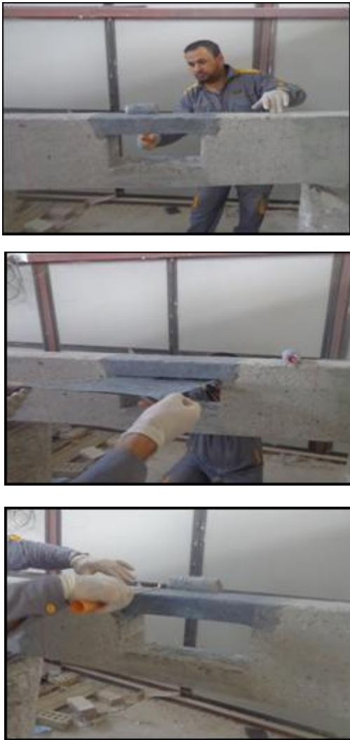
Figure (11) Cutting CFRP Sheet, Apply Epoxy on CFRP and Concrete, Placing CFRP on Concrete, and Eliminating Air Bubble.
