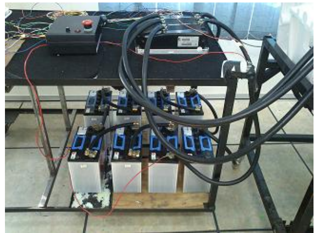
Figure 3: 8 unit 12V sealed lead acid battery connected in series to produced total of 96V
