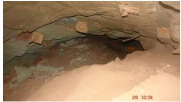
Fig. 2a. Collapsed scraper drift
