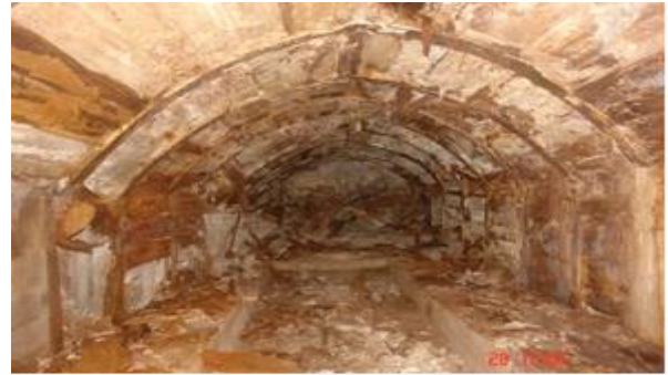
Fig. 2b. Blocked crosscut
