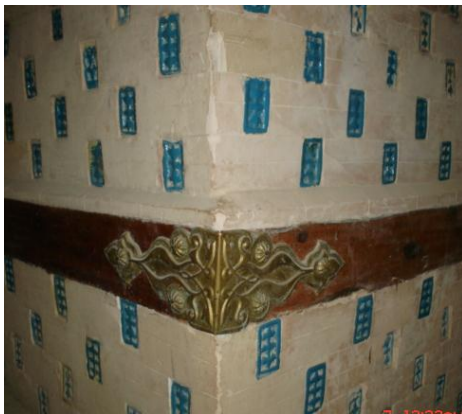
Fig. 5. Base laying type of «book-matching» and antiseismic wooden bars (reed). Kat Qala (fortress).
