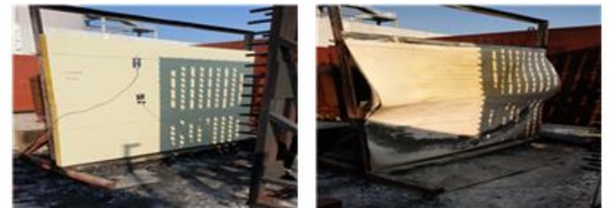
Fig. 10. Photographs of a firewall(GWS) before and after experiments.
