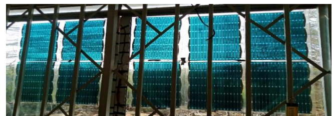
Fig. 5: Organic solar cell installed in building façade
