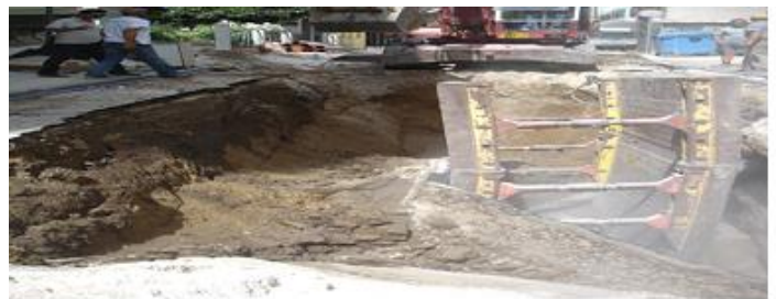
Fig. 4: Slope collapse in drainage canal, Salaminos Street, Larissa, Greece, 2010 [15].
