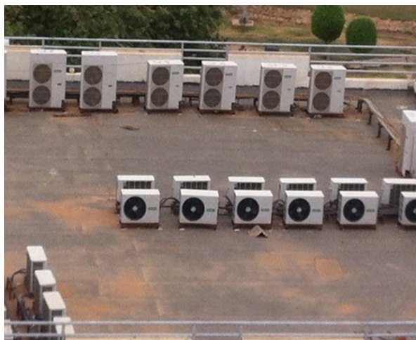
Figure 2: split cassette outdoor unit mounted on the roof of dental hospital
