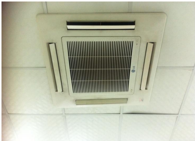
Figure 1: Split cassette indoor unit of dental hospital
