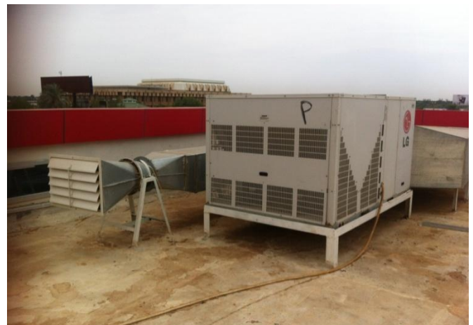
Figure 4: package unit and exhaust duct on the roof of Emergency hospital
