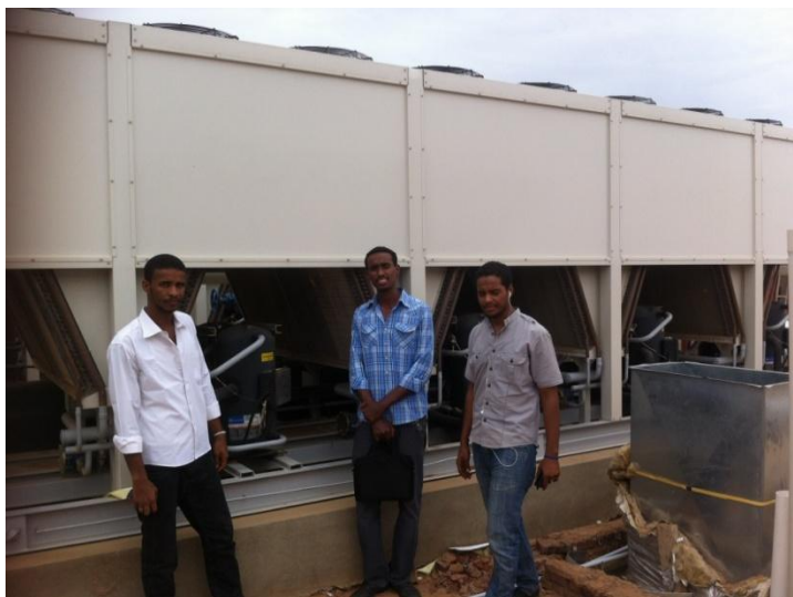
Figure 6: Air Cooled Chiller on the roof of the new specialized hospital
