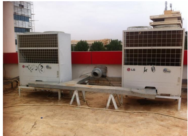
Figure 3: Ducted Split Outdoor unit on the roof of emergency hospital
