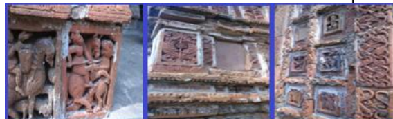
Damage of Architectures due to lack of proper managements
