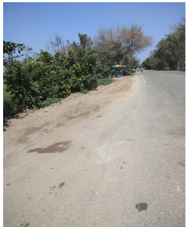
Fig 3: Shoulder deteriorated on Curve Section
