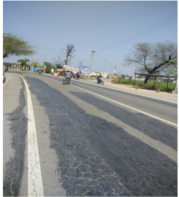
Fig 6: Deteriorated Pavement and Missing Chevron Marking for Y Junction
